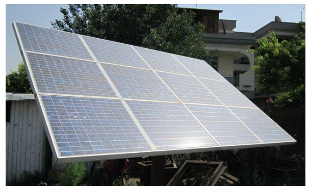
Figure 7 Fixed Solar Module System DACAAR Office Kabul
